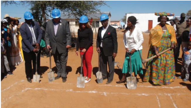
47 houses built by SDFN hand over in Otjinene and launch of construction of 11 new houses
